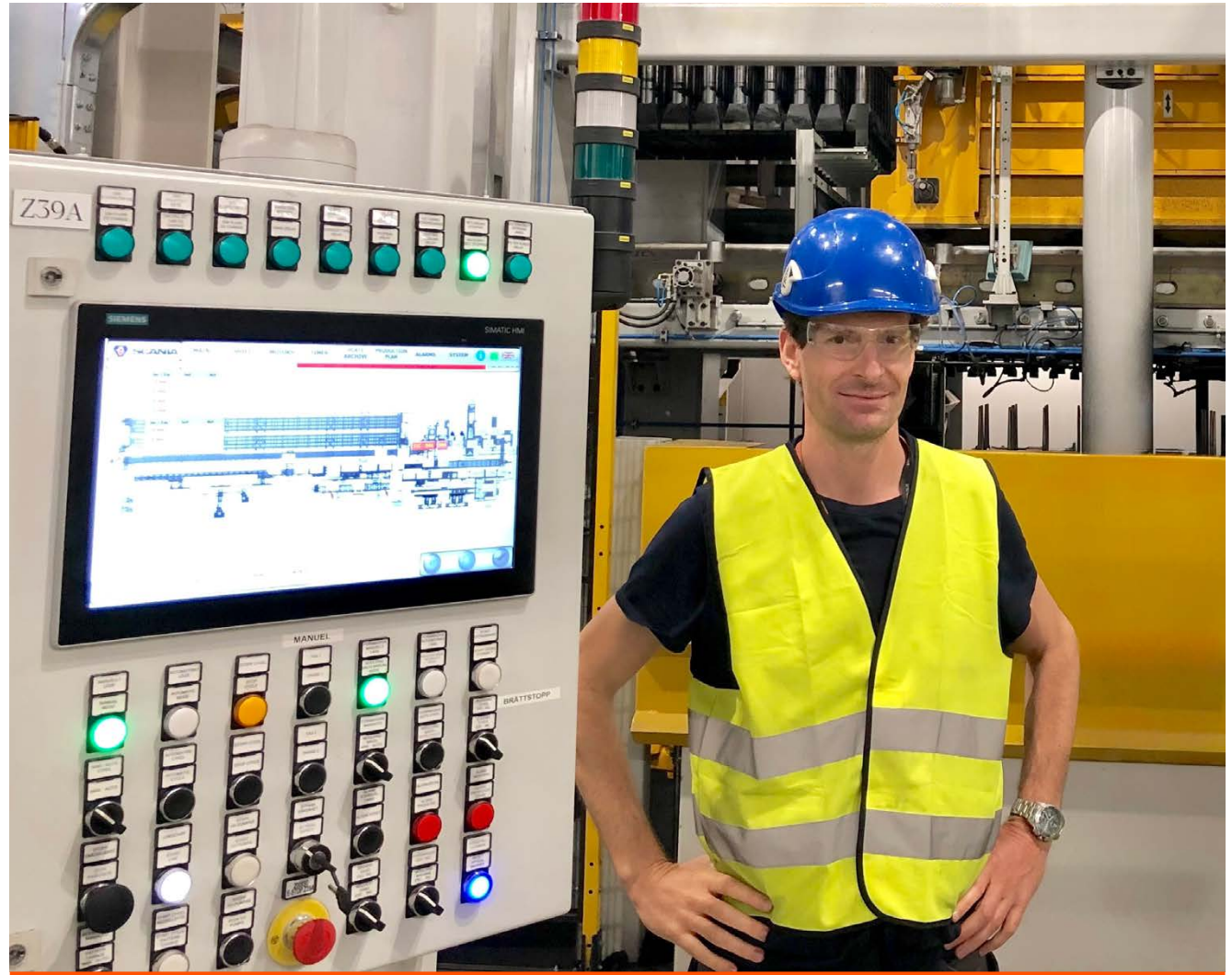
Supervisory SCADA System at the SCANIA foundry, Sweden
