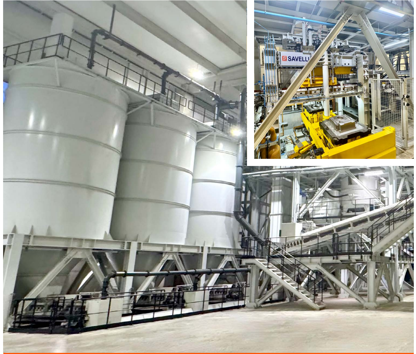
F1 Formimpress® Moulding Line with Sand Preparation and Return System at PMP Foundry, Bosnia
