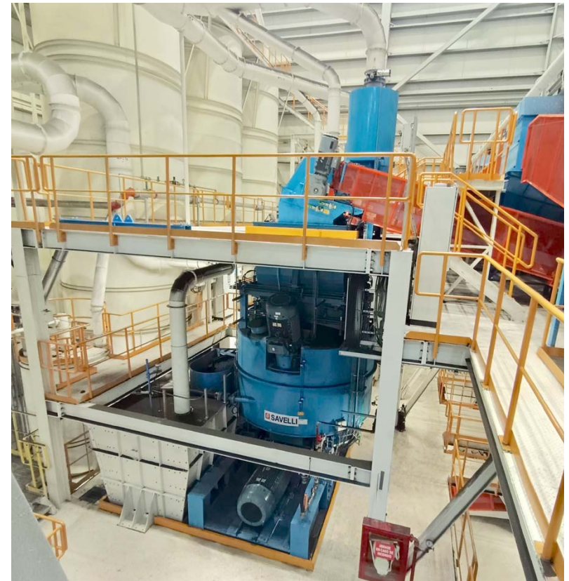
Sand Preparation Plant for the new Brembo foundry, Mexico
